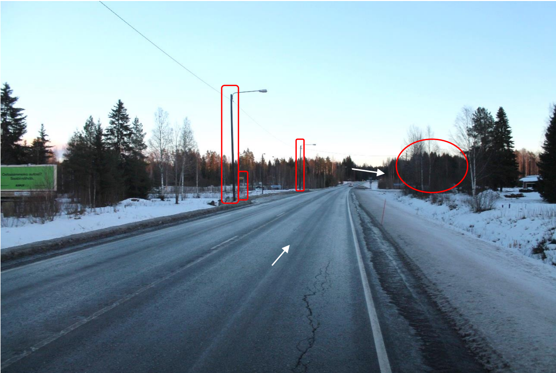
Pos 1/Pic 1. Turning from road 11 toward road 2492. https://maps.app.goo.gl/tyKyKsinutRNpEwW6 Marked sign and lamp posts need to be removed. Marked trees need to cut on private property.
